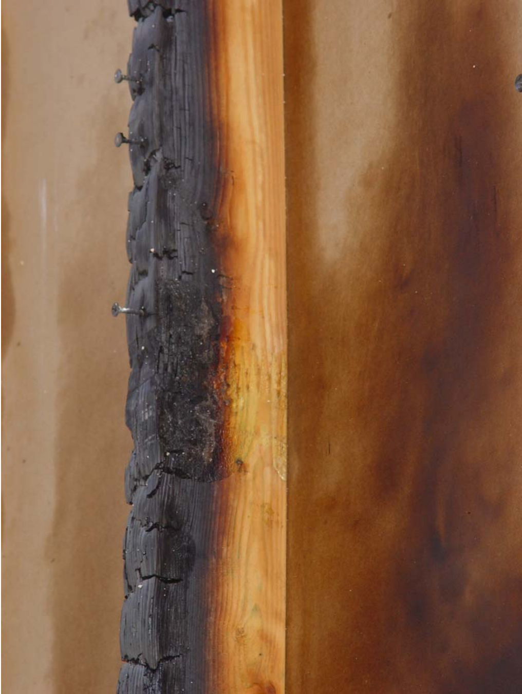
Charred stud at finger-joint
